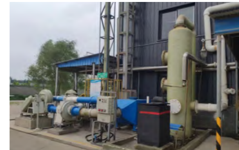
Before retrofitting: Activated carbon adsorption device + Alkali spray absorption
