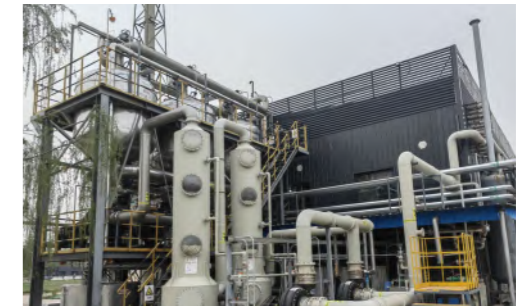
After retrofitting: Alkali spray absorption + Water spray absorption + Resin adsorption
